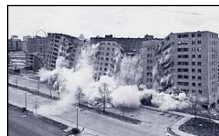
Destruction of one of the Pruitt-Igoe buildings. Photo courtesy of the St. Louis Post-Dispatch.
